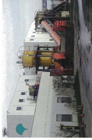
Soil Improvement Plant
